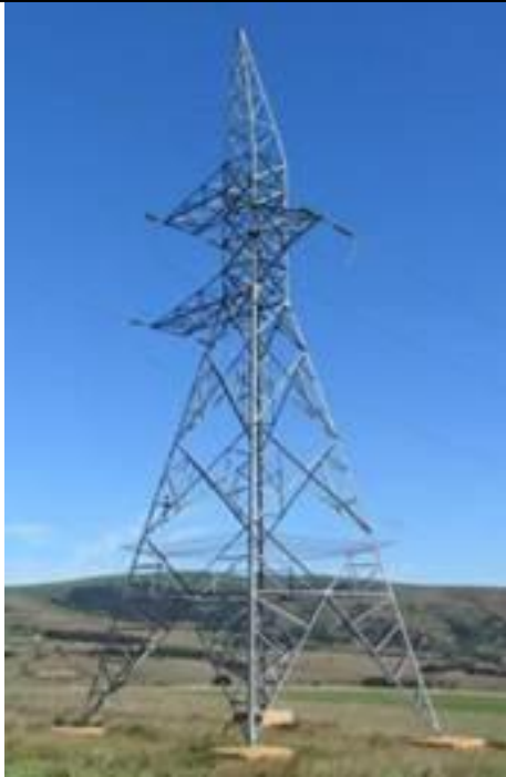
Figure 3: Self-supporting strain tower (255D)
