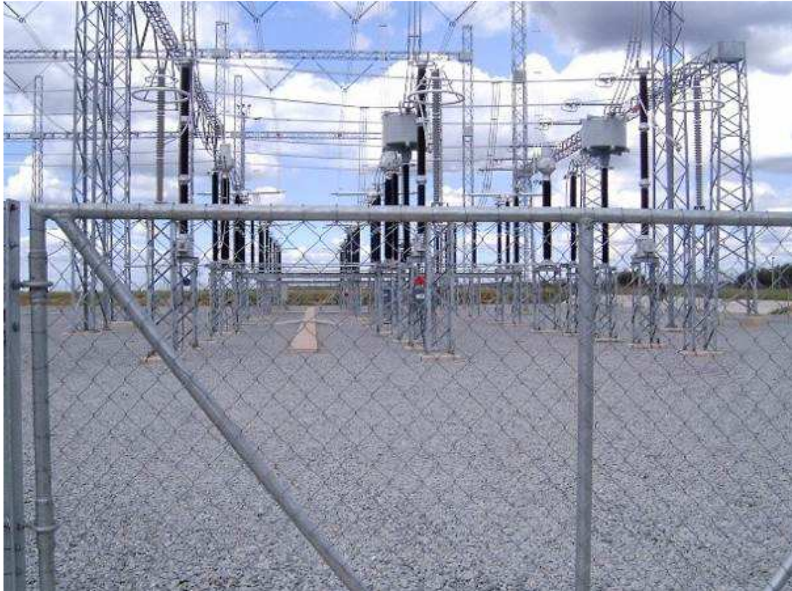
Picture depicts a typical Substation facility
