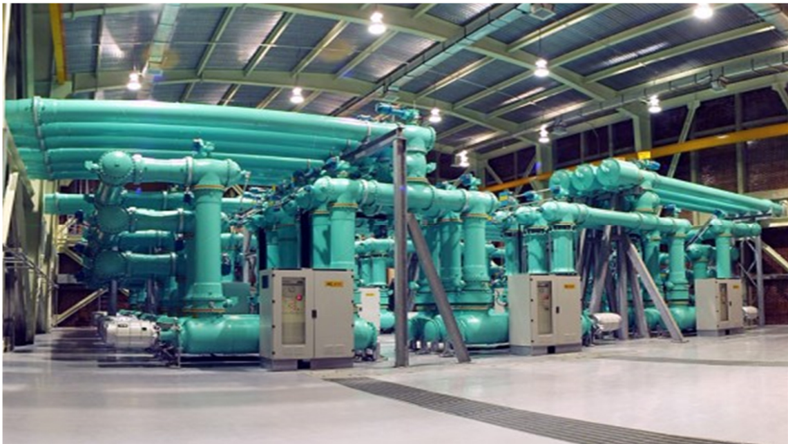
Figure 3:2 GIS is totally enclosed within a building
