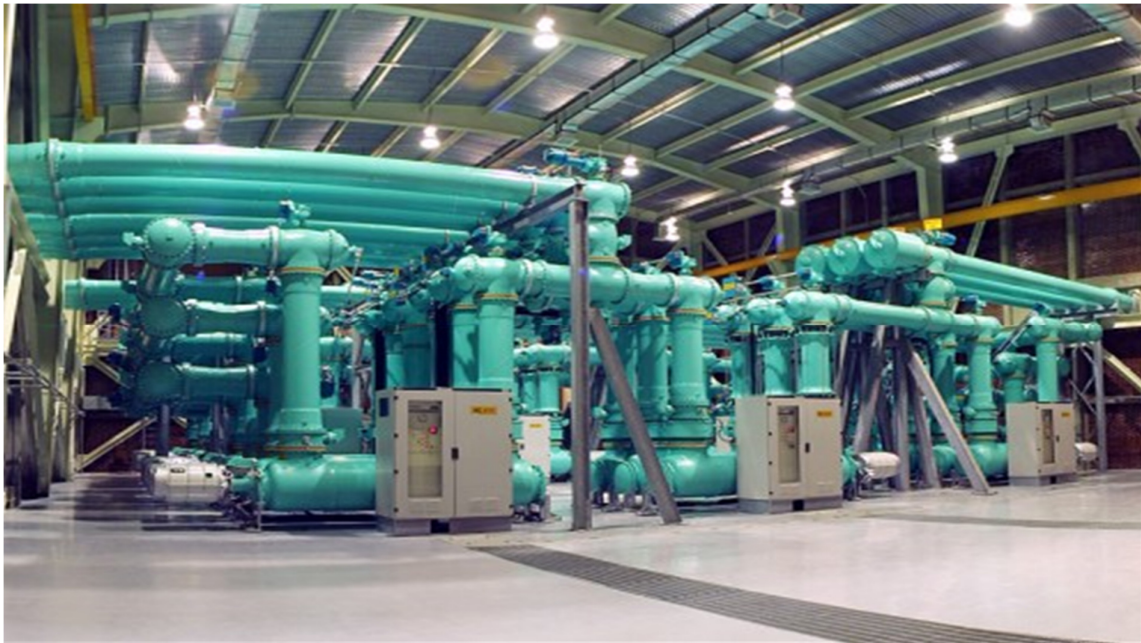
Figure 3:2 GIS is totally enclosed within a building
