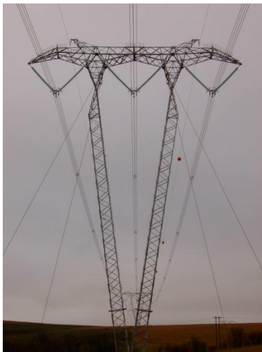
Guyed V suspension tower
